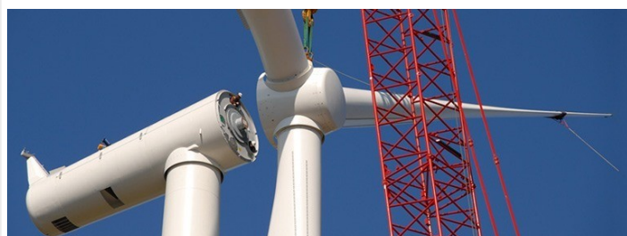
Workers build a turbine for the Maine Renewable Energy Interconnect project. Source: Maine Renewable Energy Interconnect
